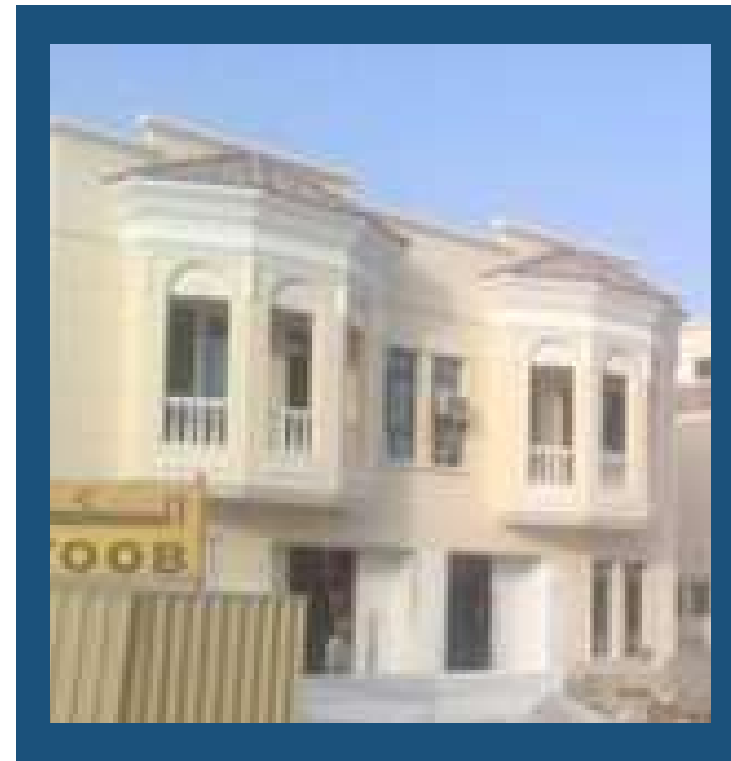
Project: 25 NOS TWIN HOUSE GROUND + ONE VILLAS Location: Plot No. 643-7692, 643- 7696, 643-7697&643-7698 at Wadi Al Safa-2, Dubai-U.A.E. CLIENT: MR. MOHAMMAD HABIB MOHAMMAD HABIB AL REDAH CONSULTANT: GULF ENGINEERING
